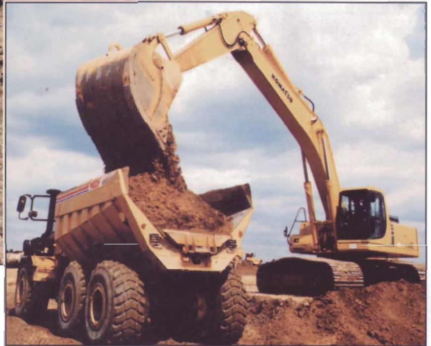
The operator of a Komatsu excavator loads a Moxy articulated truck at a Mount Construction jobsite.
