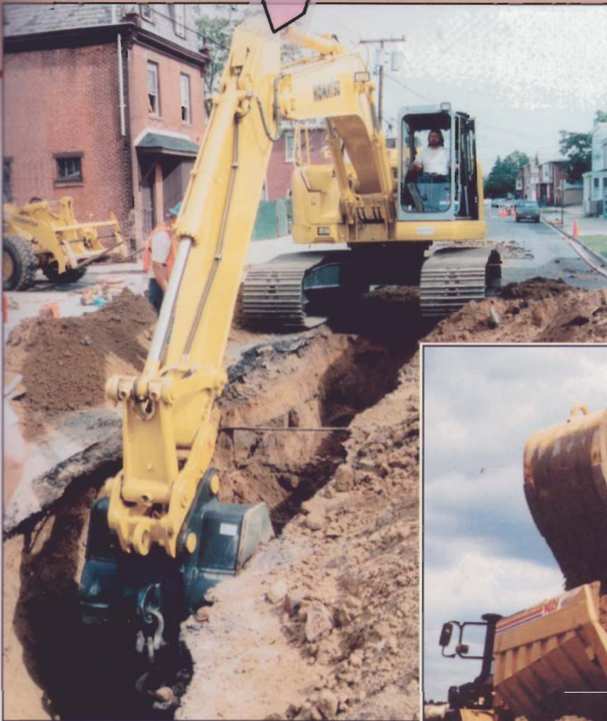
Mount Construction added this PC228USLC-2 excavator to its expanding fleet of Komatsu equipment to help crews work in confined and congested urban areas. The "short-tail-swing" excavator is pictured at left on a recent underground utility project in Gloucester City, New Jersey.
